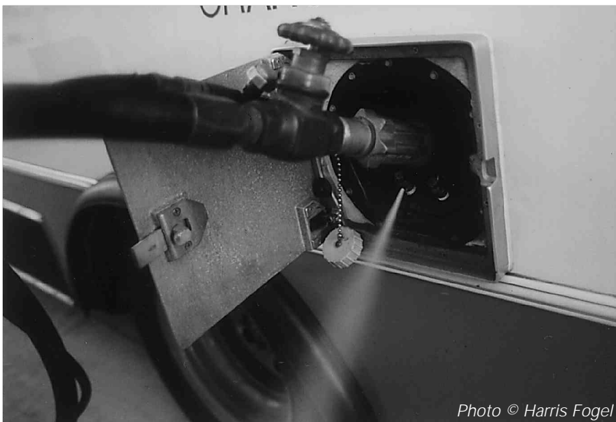
22-3 Liquid level gauge venting vaporizing liquid; 80% of capacity, tank full.
