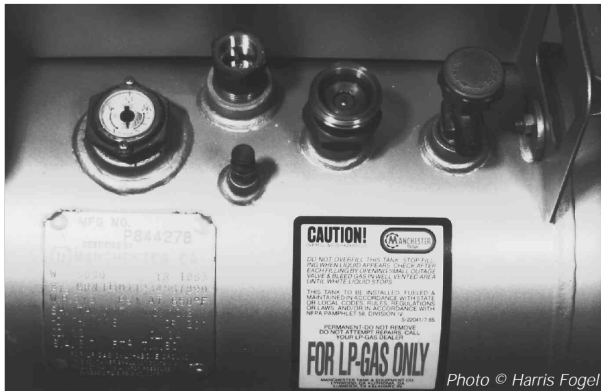
13-1 Typical tank valve and gauge layout – plumbing not connected.
