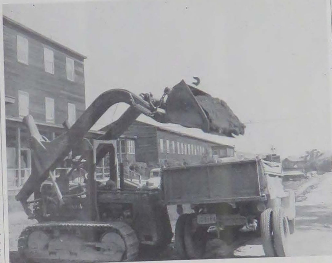
A mechanical "super-shovel" is seen as it fills a dump-truck—one step in the repair work, now in progress on the roads at Oak Knoll.
